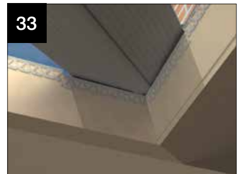
33 Where plasterboard intersects with the valley undercladding it should be notched to fit and fitted with LVPT250/1 PVCu plasterboard trim.
