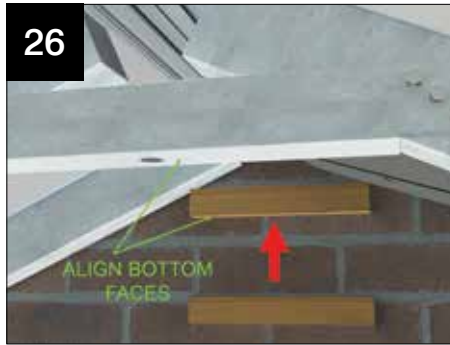
26 Fit a length of timber batten to the host wall, ensuring that its underside lines through with the underside of the struts (LVTS001/LVTS002). This will provide a fixing point for the ridge board fitted in the next step.
