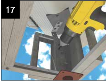
FIT THE STRAP CHA018 USING M4x13 SELF DRILL SCREWS, to the valley corner infill panel and the valley fixing bracket. It may be necessary to bend CHA008 to suit.
