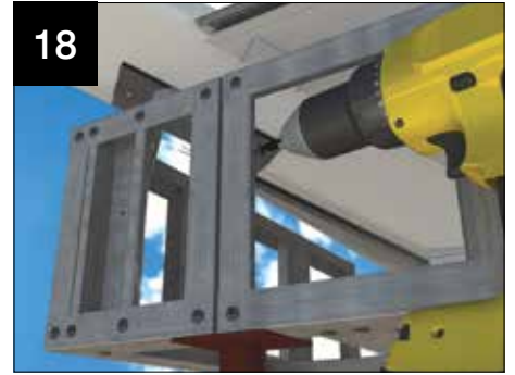
Fit the vertical frames. Fix the frames into the valley corner infill and the horizontal frames.
