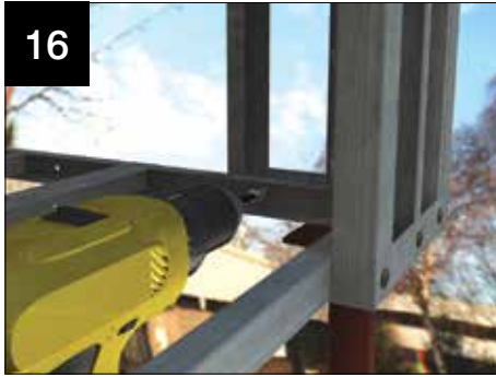
Fit the valley corner infill panel to the horizontal frame, level up and secure to the valley plate.
